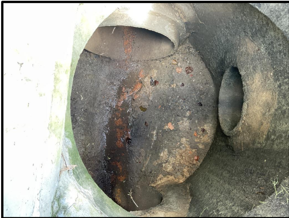
Photo #2: Minor road grit accumulation present
