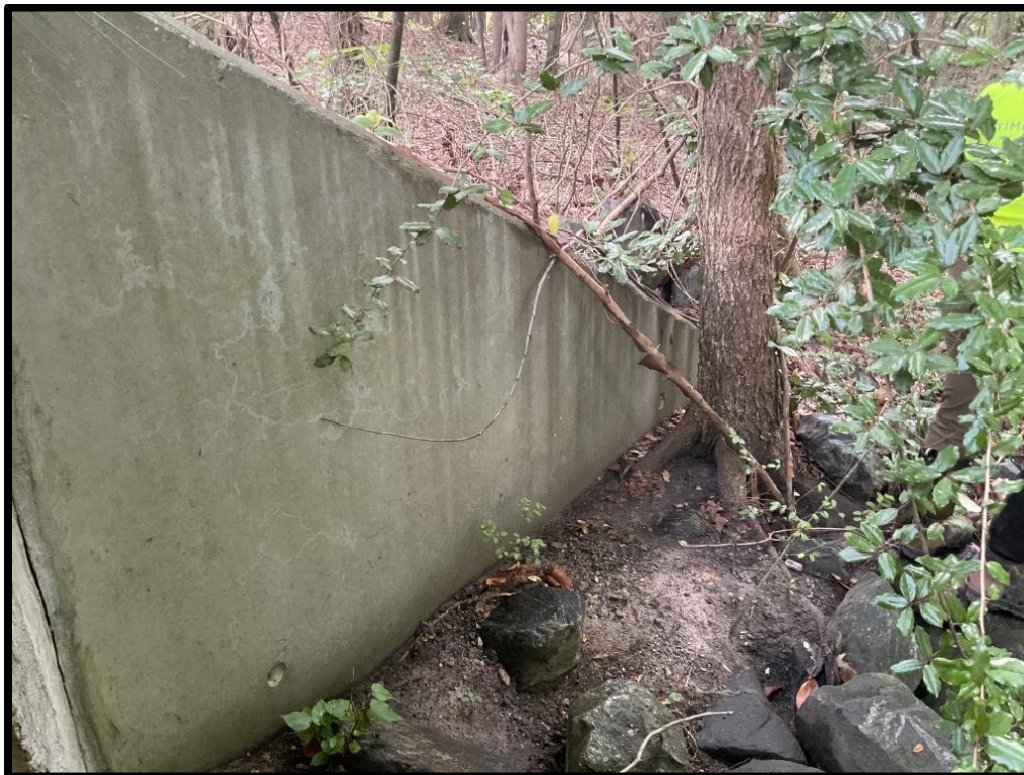
Photo #4: Tree growing into headwall
