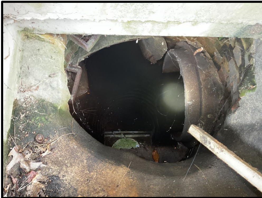
Photo #2: Standing water present
