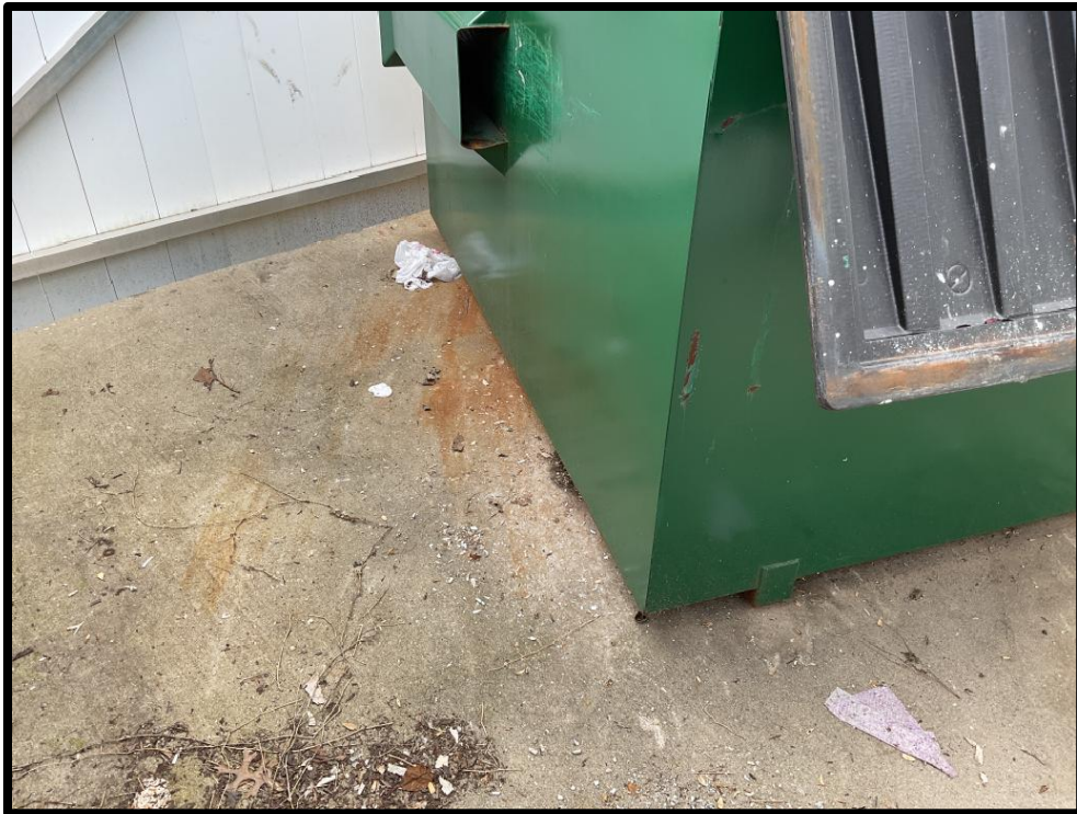
Photo #1: Rust present under dumpster
