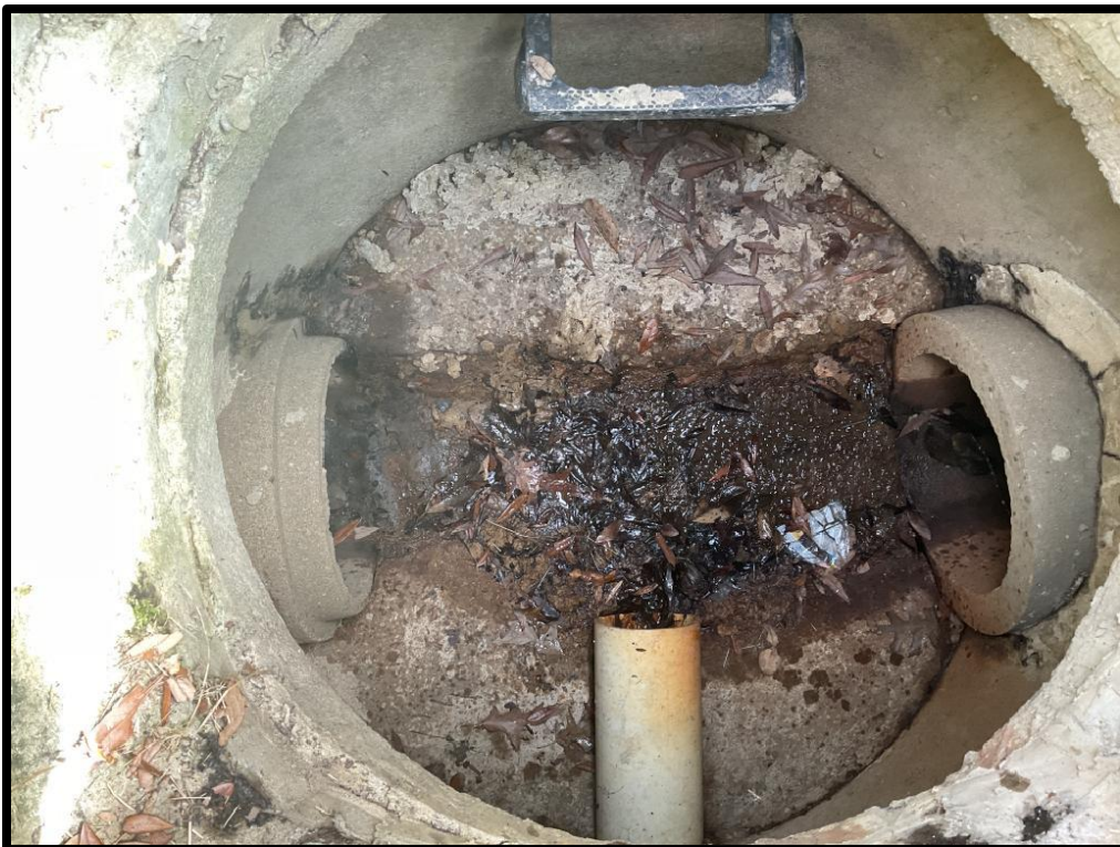
Photo #4: Some debris accumulation present in underdrain outlet pipe
