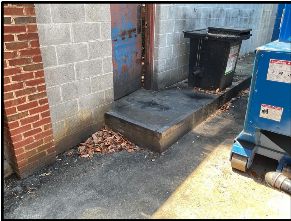
Photo #1: Stains from grease trap
