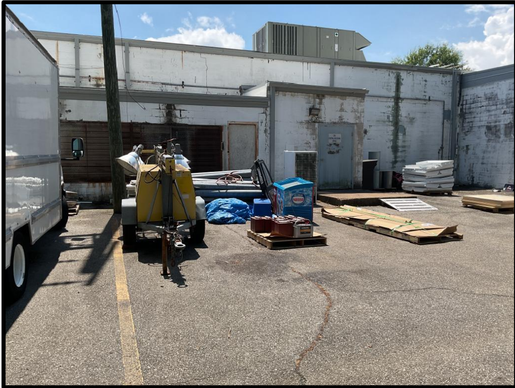
Photo #3: Uncovered materials storage area
