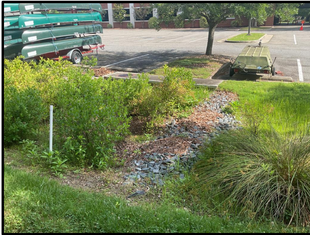
Photo #5: Some debris accumulation present in eastern check dam
