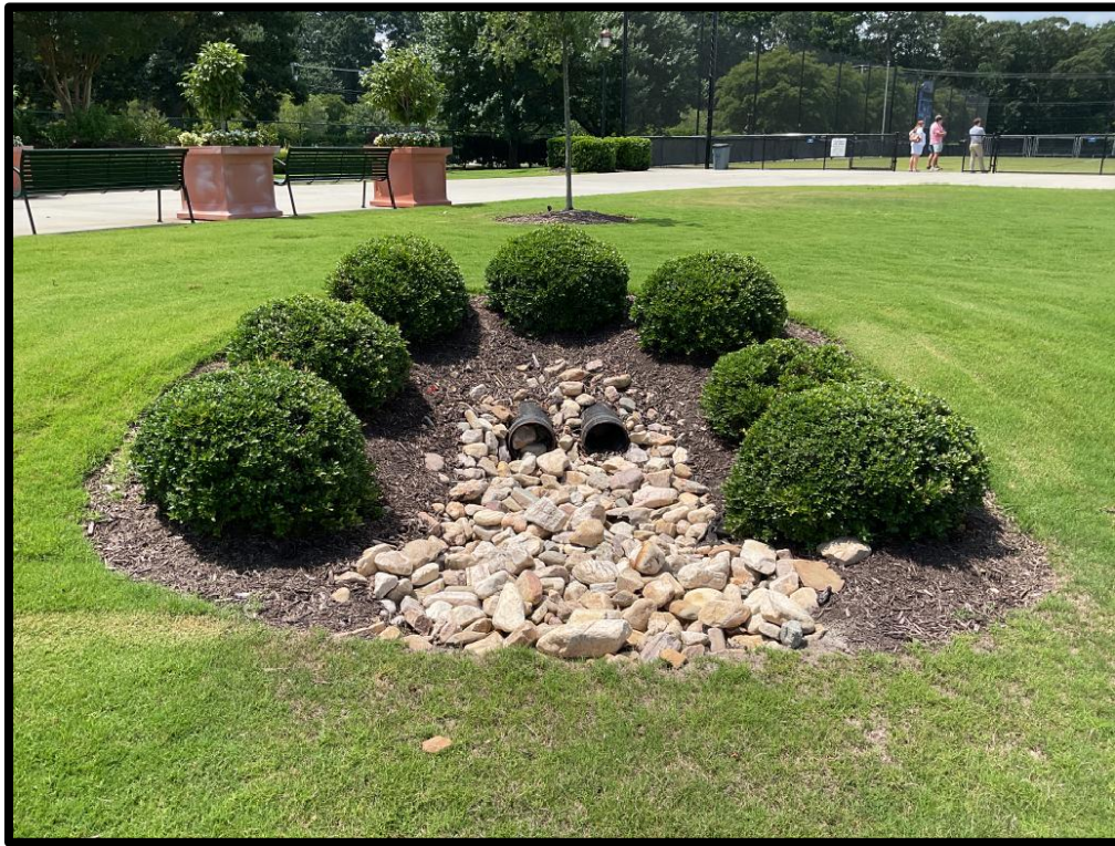
Photo #5: Stone present in southwest inlet pipe
