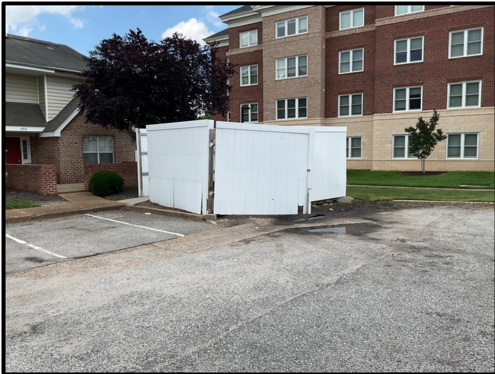
Photo #2: Sediment accumulation outside of receptacle area
