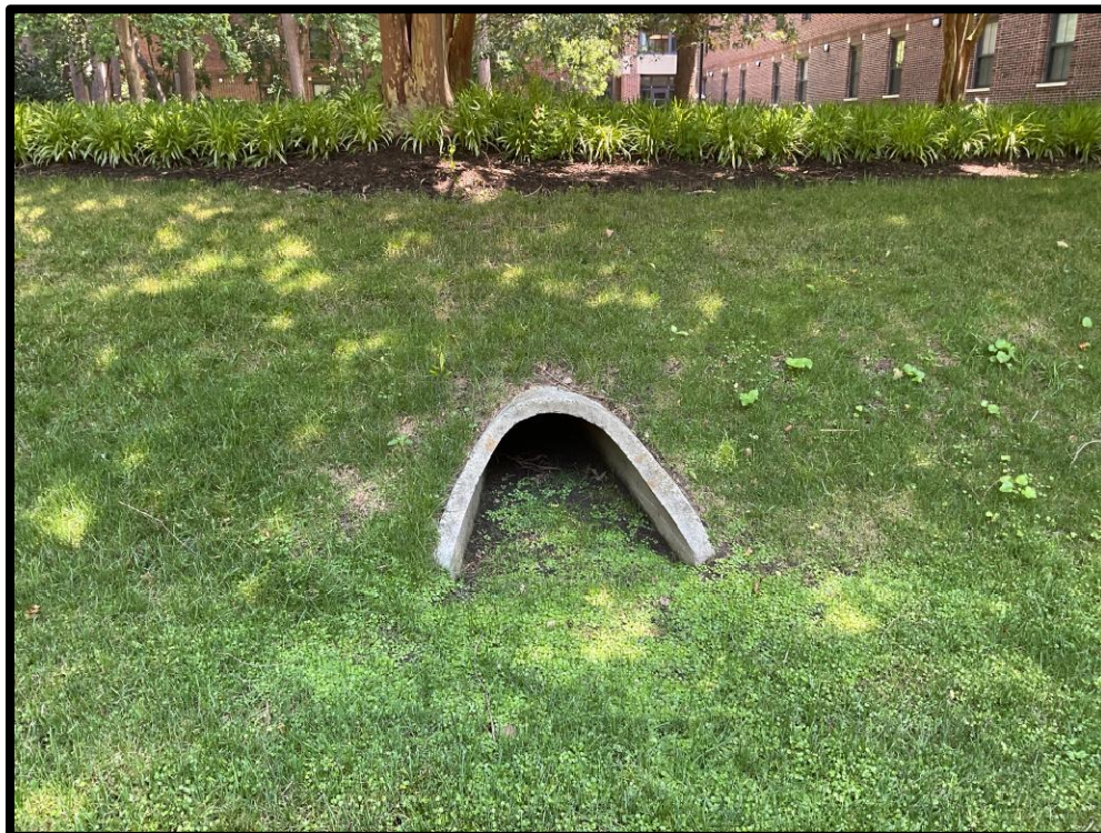
Photo #6: Sediment and vegetation accumulation present in eastern inlet pipe and protection
