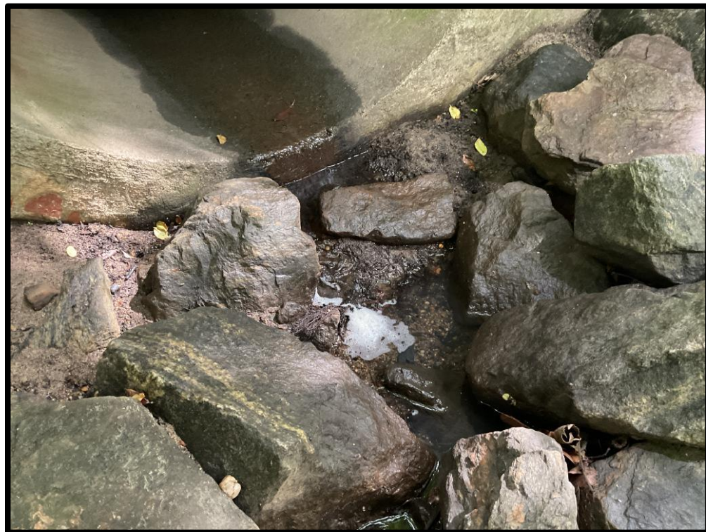
Photo #2: Ground water present
