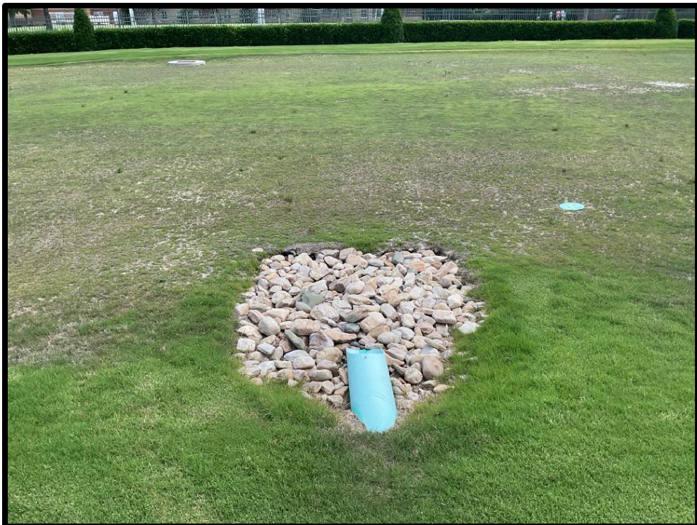
Photo #4: Some scour present around western inlet protection
