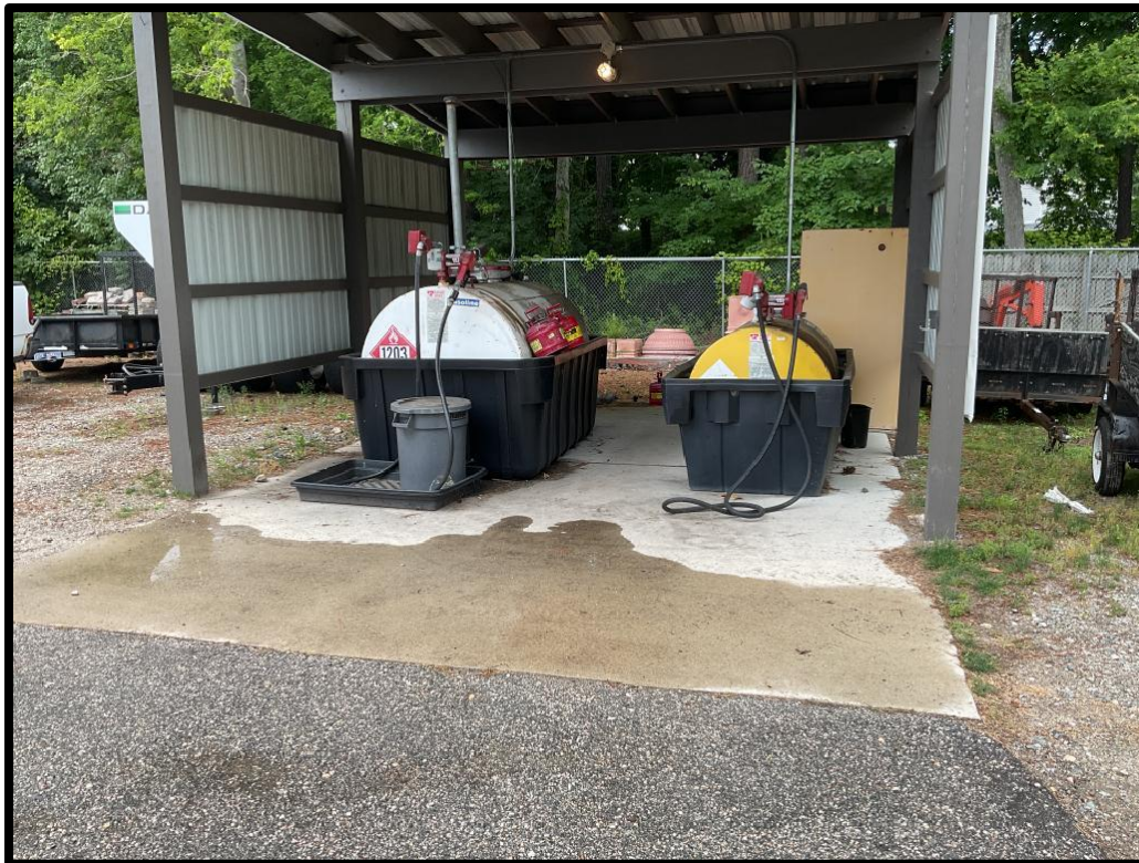
Photo #10: Covered fueling area with secondary containment and spill kit
