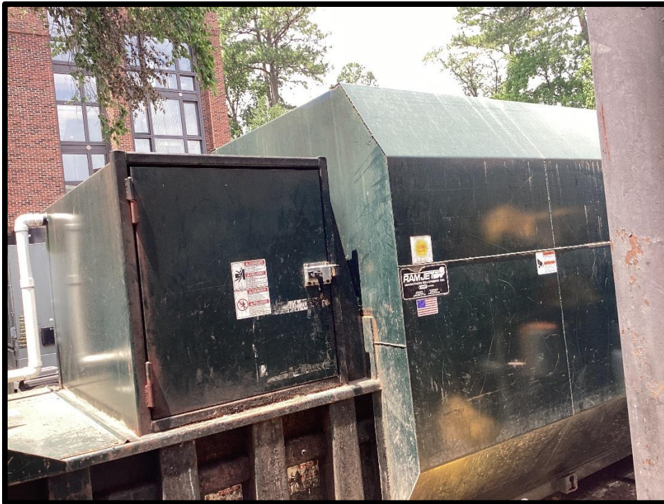
Photo #1: Trash compactor
