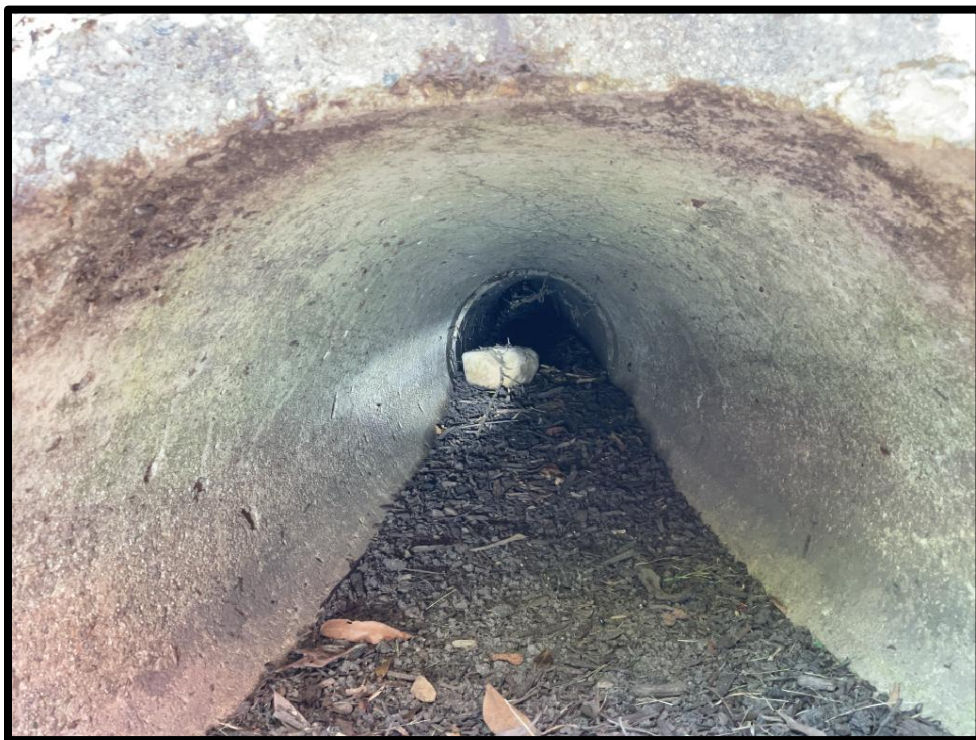
Photo #2: Sediment and debris accumulation present in southern inlet
