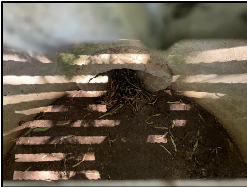
Photo #8: Some sediment accumulation and debris present in outlet structure
