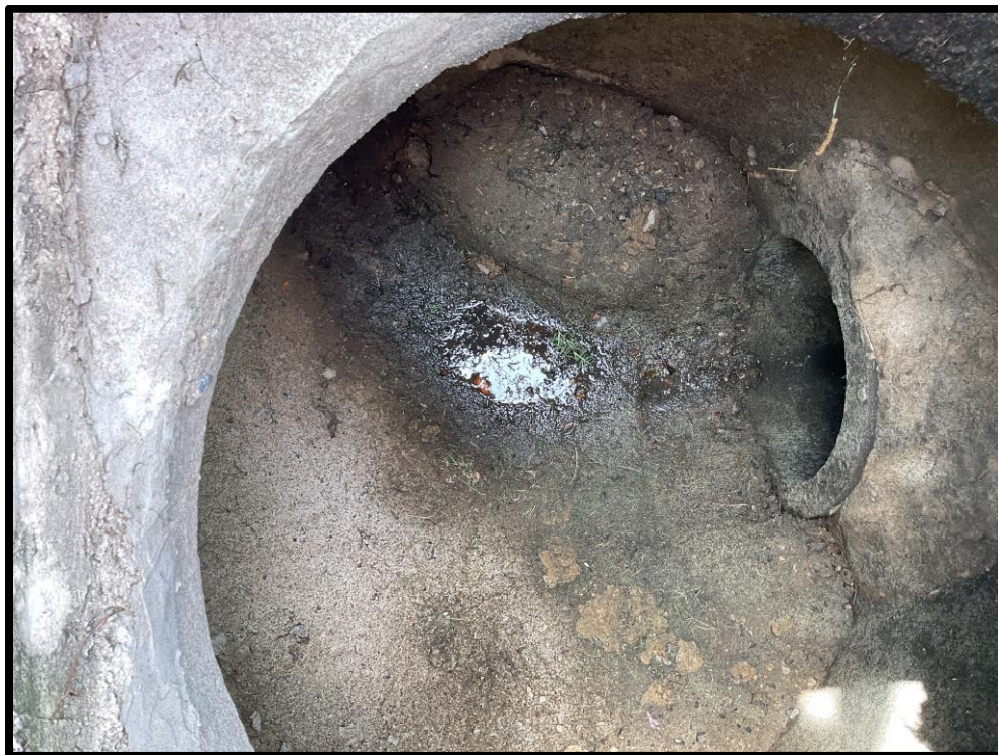
Photo #2: Minor sediment accumulation present
