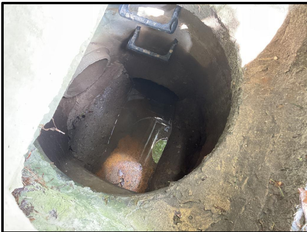
Photo #2: Sediment accumulation and backwater present
