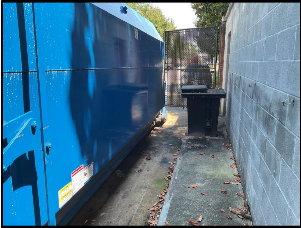
Photo #3: Staining present under trash compactor
