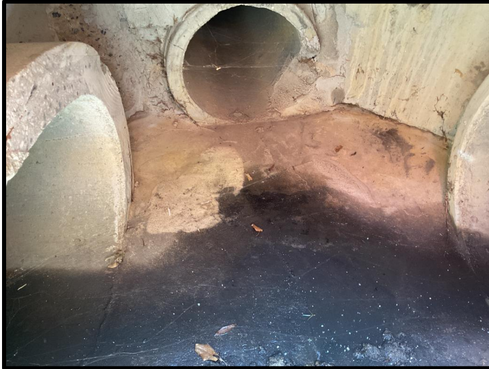
Photo #3: Downstream outfall pipe, some sediment accumulation present
