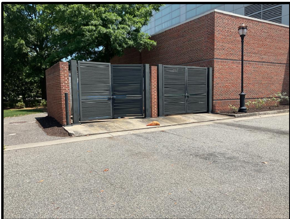
Photo #2: Sand bag and stains present near receptacle area
