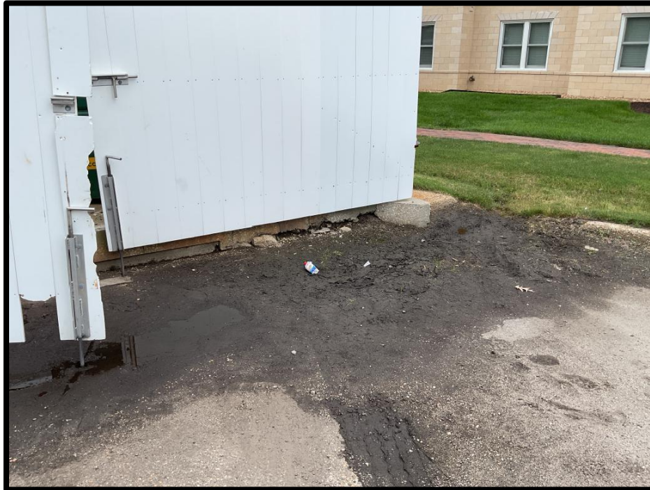
Photo #3: Significant sediment accumulation outside of receptacle area, clogging inlet
