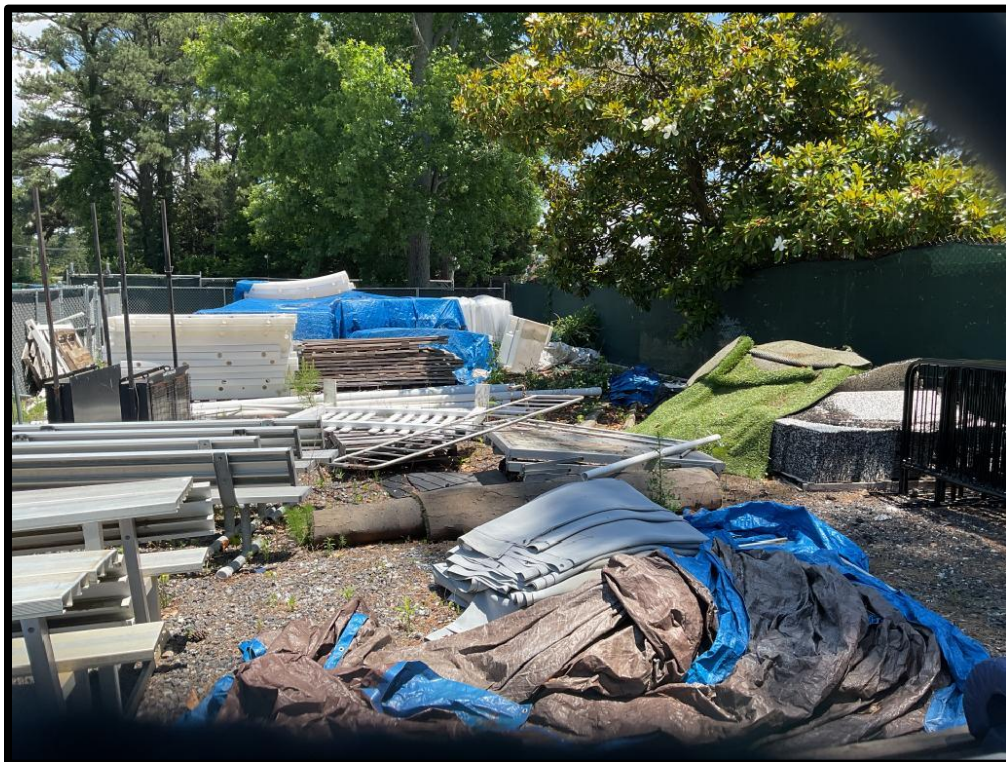
Photo #6: Uncovered materials storage area
