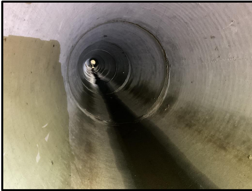
Photo #3: Pipe is disjunct
