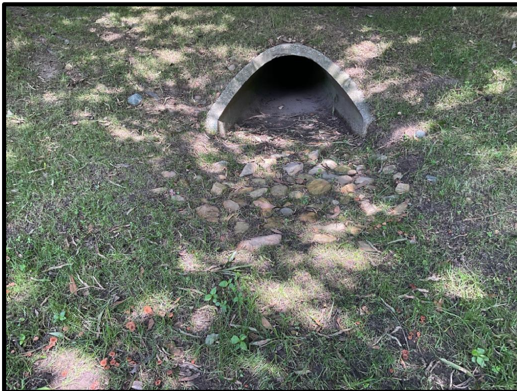
Photo #4: Sediment accumulation present in northern inlet protection
