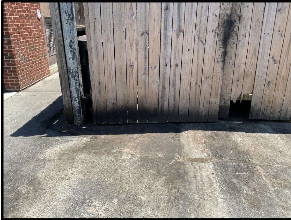
Photo #5: Stains from trash compactor present
