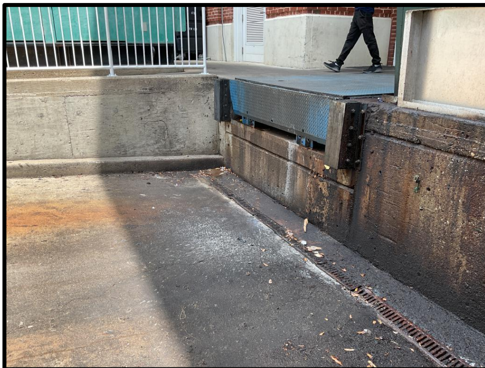
Photo #2: Debris accumulation near trench drain
