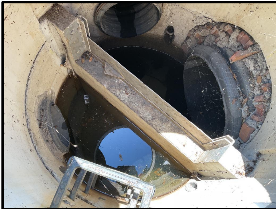
Photo #2: Some debris accumulation present in northern structure
