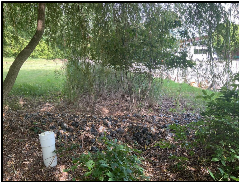
Photo #6: Some debris accumulation present in western check dam
