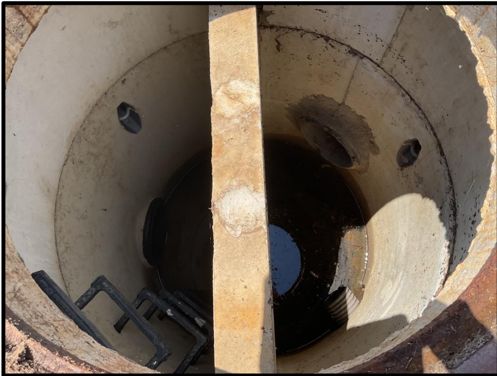
Photo #3: Some debris accumulation present in southern structure
