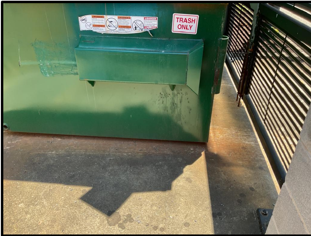
Photo #3: Rust stains present under dumpster
