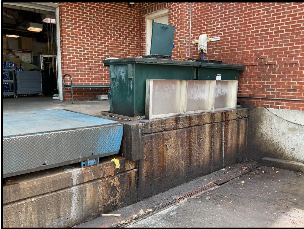
Photo #3: Grease traps appear to be draining into trench drain
