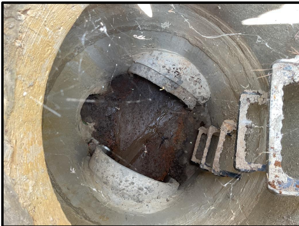
Photo #2: Significant sediment accumulation present
