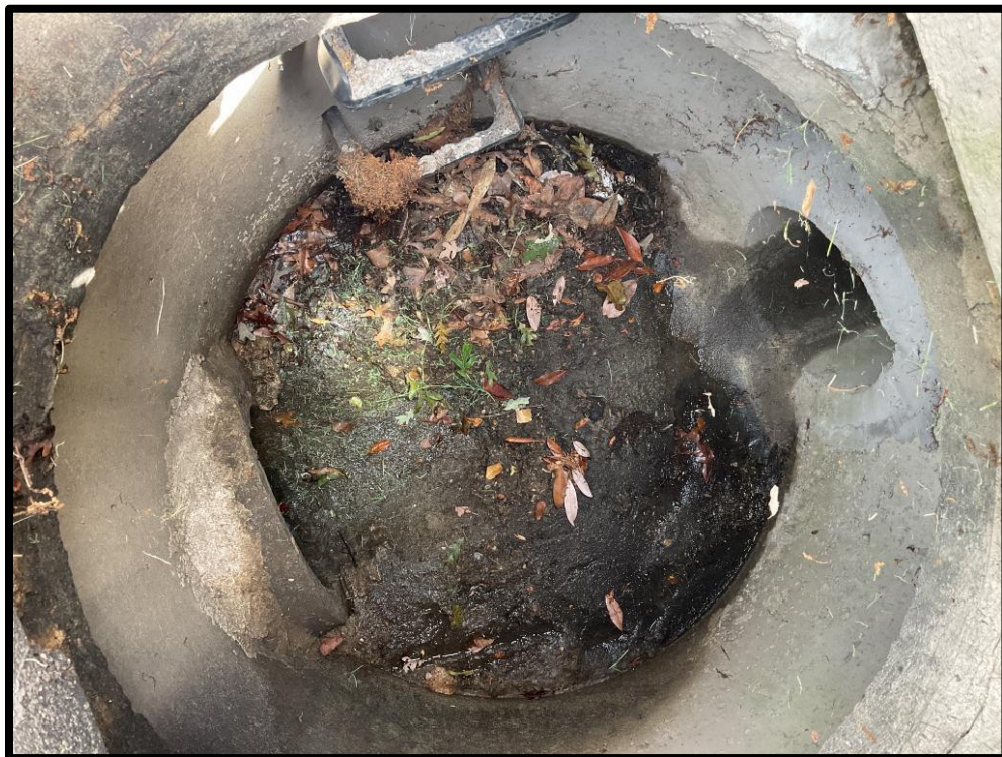
Photo #2: Some sediment and debris accumulation present
