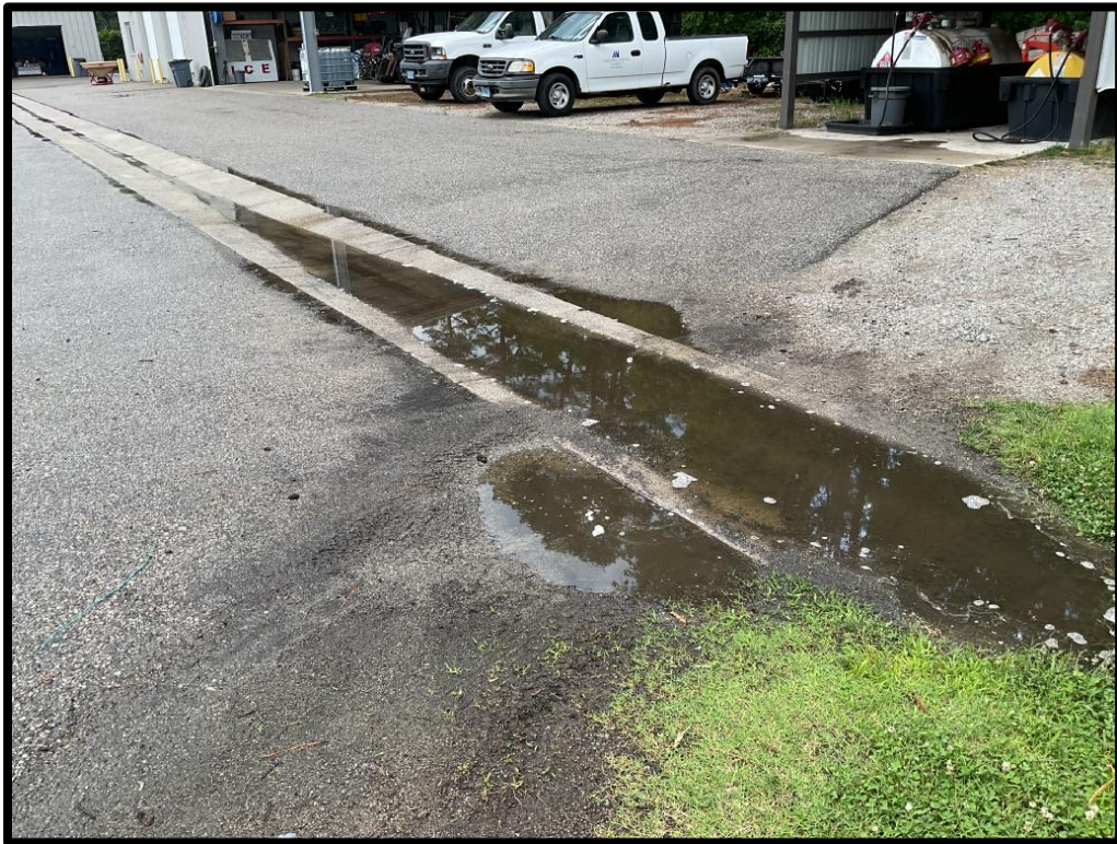
Photo #13: Suds observed in stormwater conveyance channel
