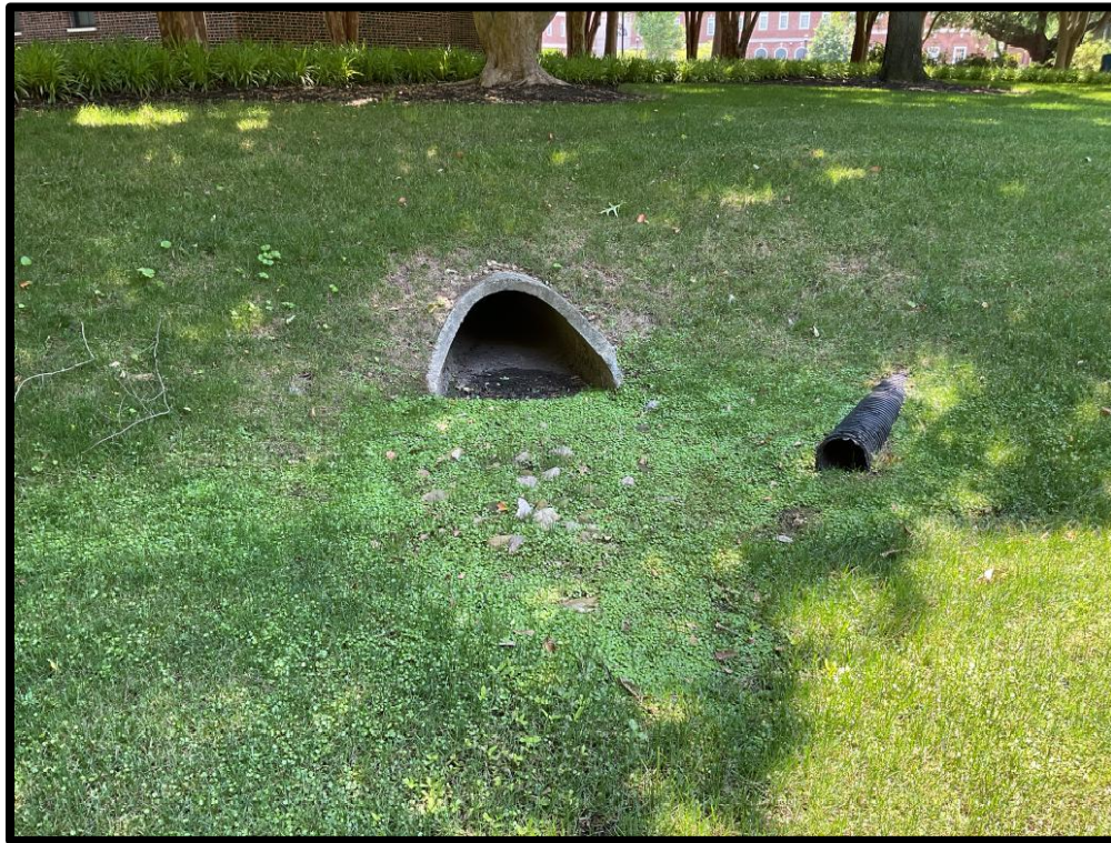
Photo #5: Sediment and vegetation accumulation present in southeastern inlet protection
