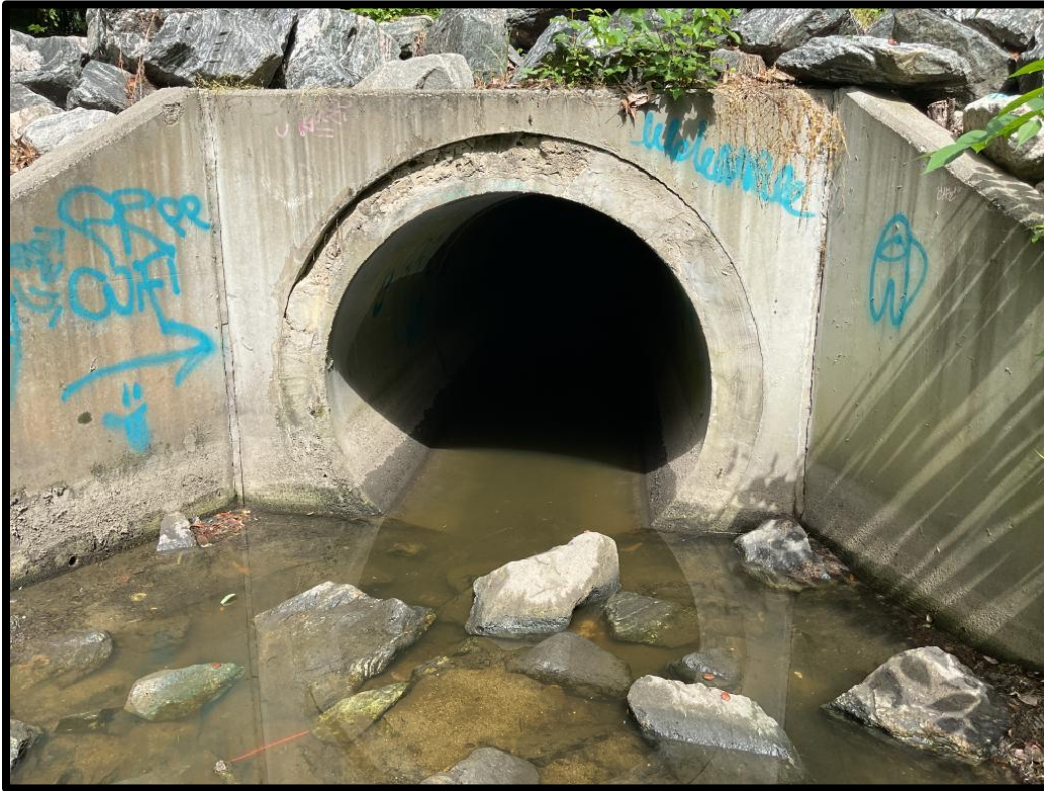
Photo #3: Some flow from upstream, backwater present in pipe due to receiving channel conditions
