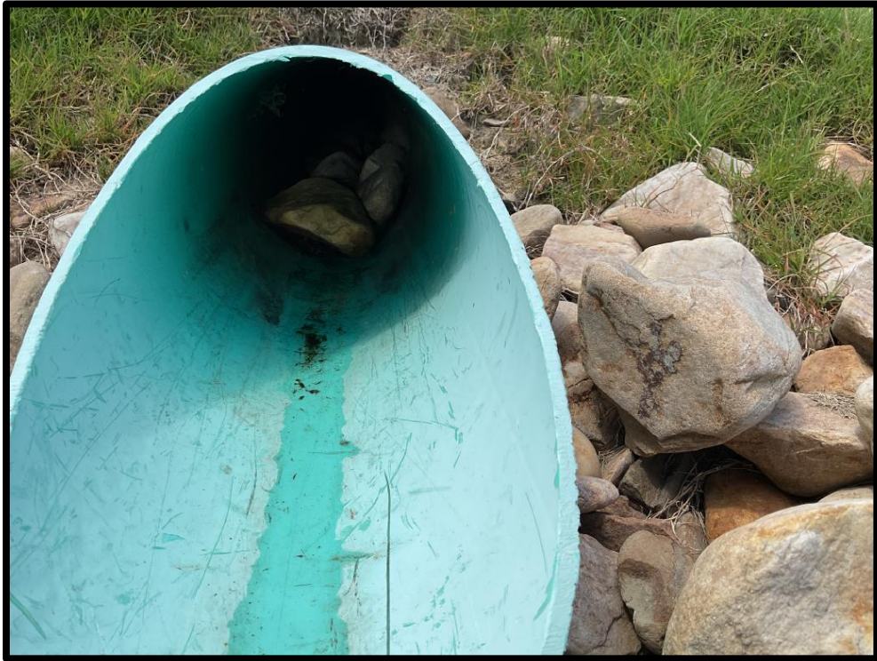
Photo #3: Stone present in western inlet pipe
