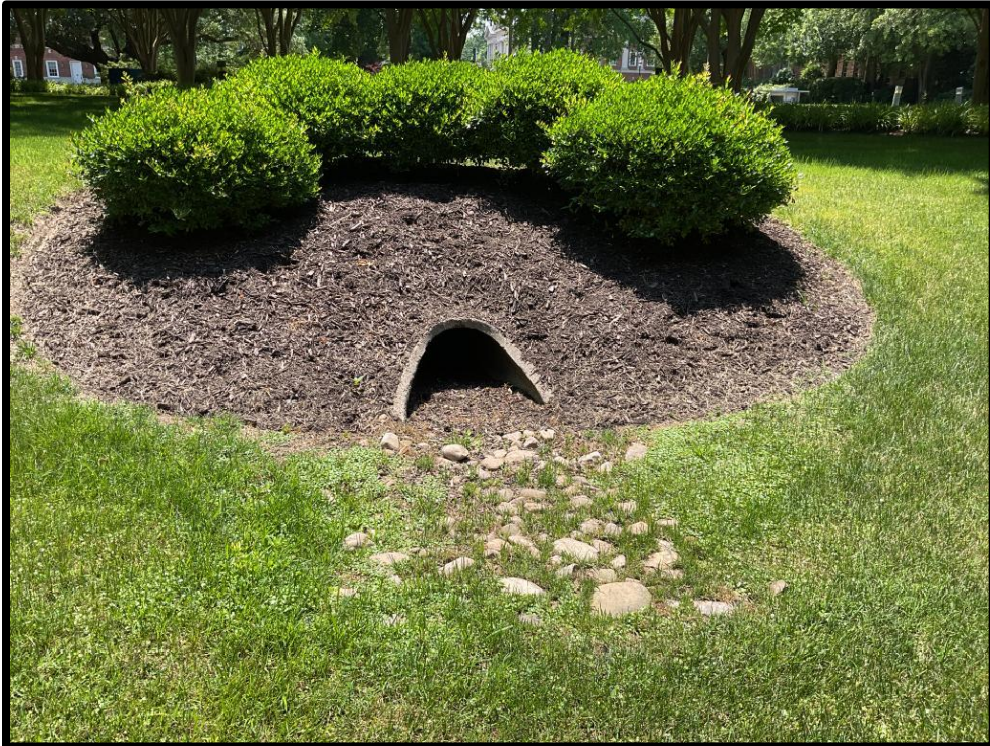
Photo #3: Sediment and vegetation accumulation present in southern inlet pipe and protection
