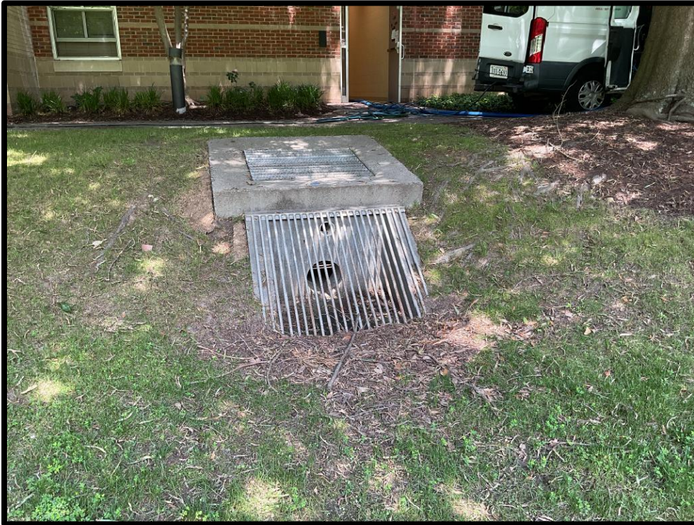
Photo #7: Minor debris accumulation present in outlet trash rack, some denuded areas around outlet structure
