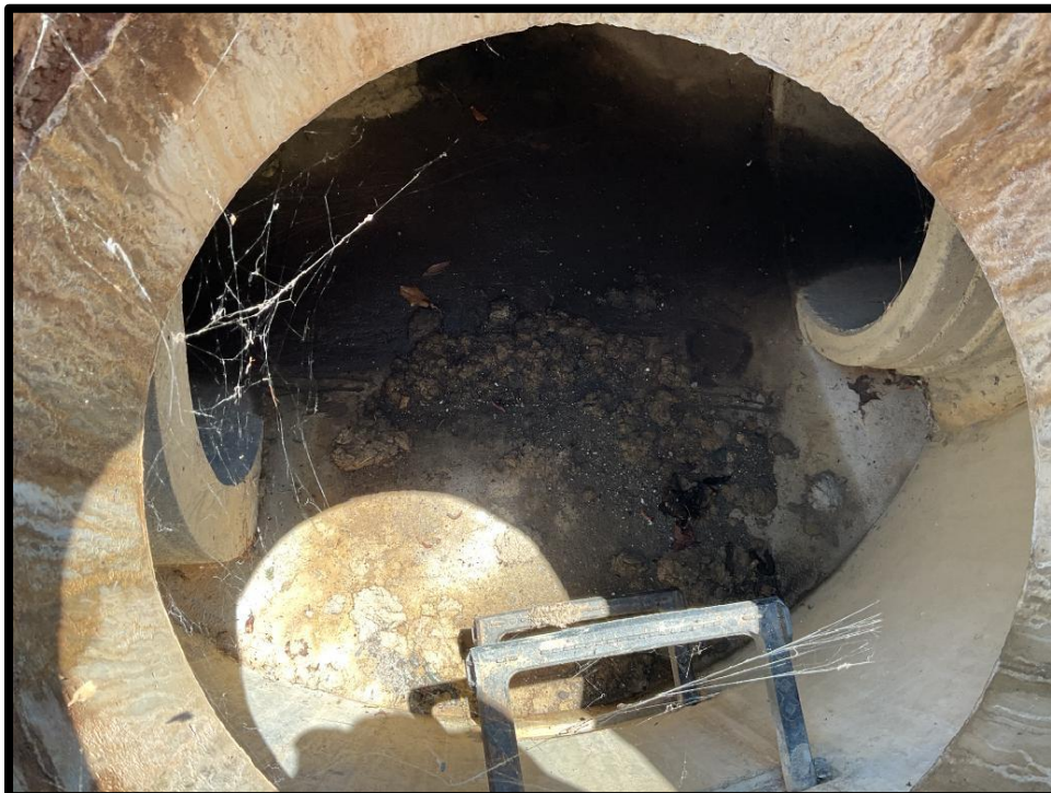
Photo #2: Upstream outfall pipe, some road grit accumulation present
