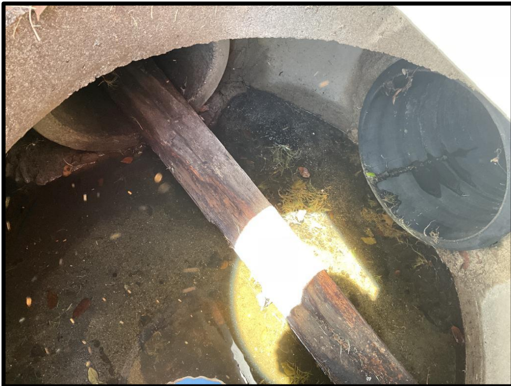
Photo #4: Some debris accumulation present in upstream inlet structure
