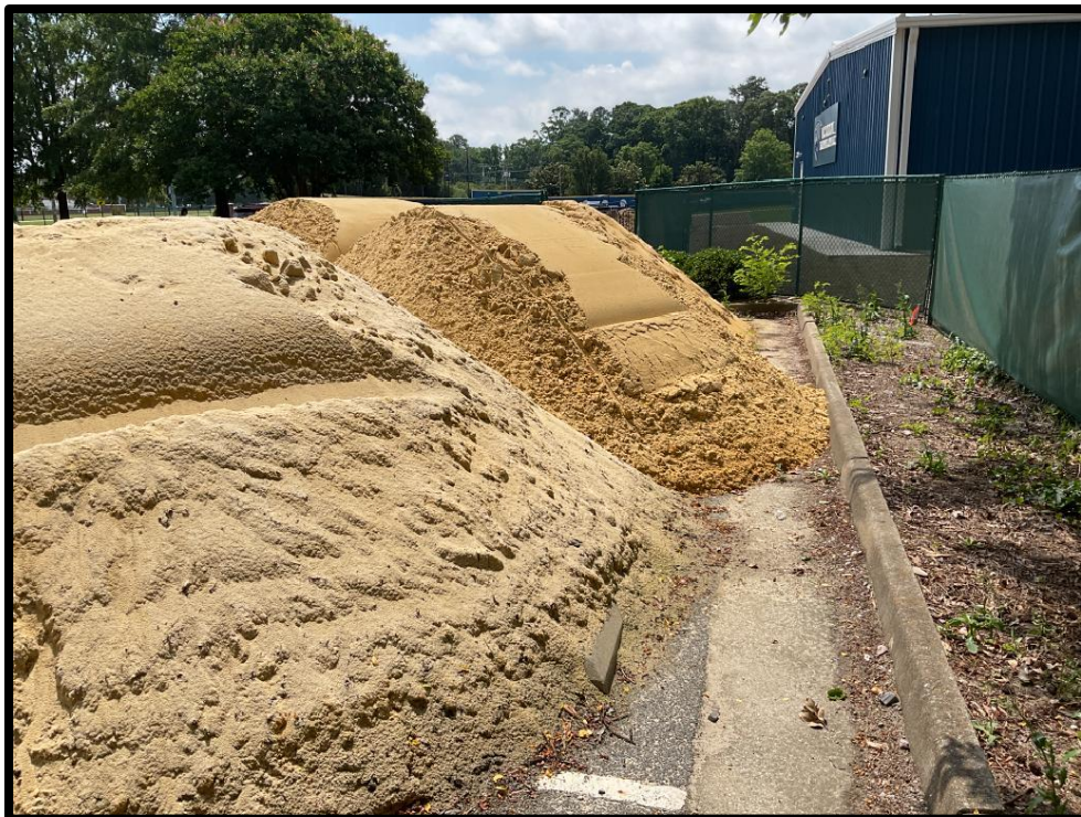
Photo #4: Back side of uncovered stockpiles
