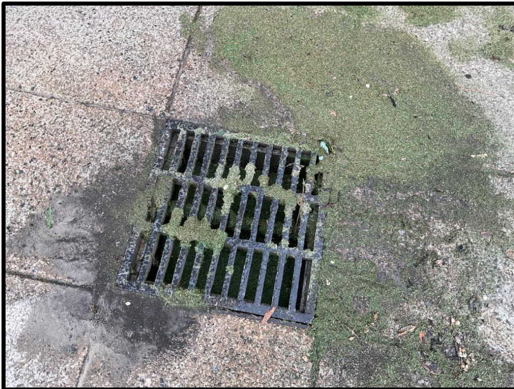
Photo #6: Grass clippings and road grit present at vehicle wash station inlet grate
