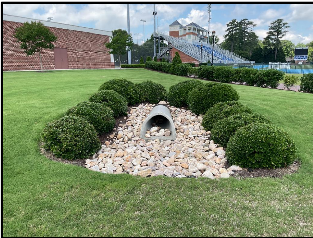
Photo #6: Stone present in northern inlet pipe
